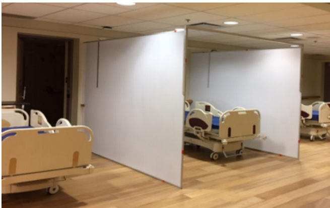
Installation of partition walls to expand ICU capacity in local hospital in Canada
